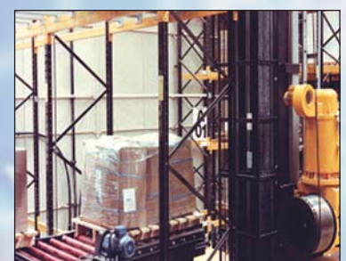
Interfacing with Warehouse Cranes
